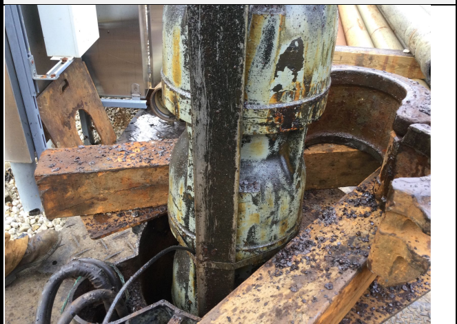
3. Cable guard intact
