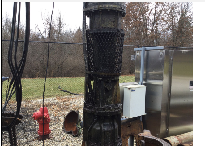
4. Cable guarded properly
