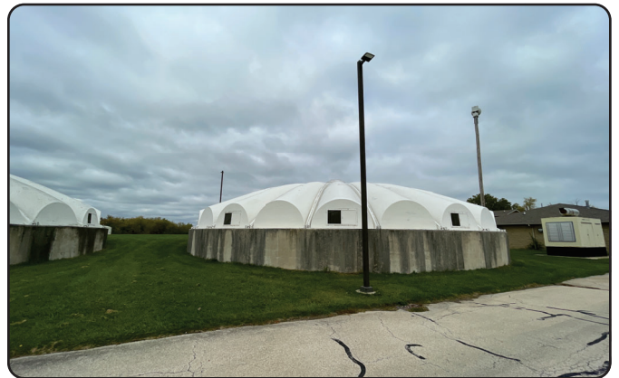
O'Carroll to replace drivers and fuses for all blinking fixtures at the Wastewater facility; this is an issue with incompatible LED drivers
