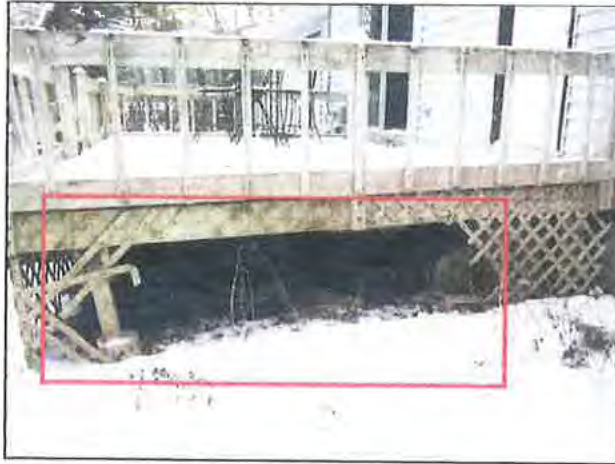
1.5 Debris should be removed
